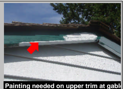
Painting needed on upper trim at gable.
