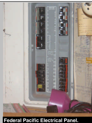
Federal Pacific Electrical Panel.
