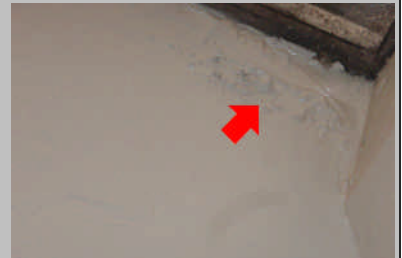
Past leakage at corner of skylight.
