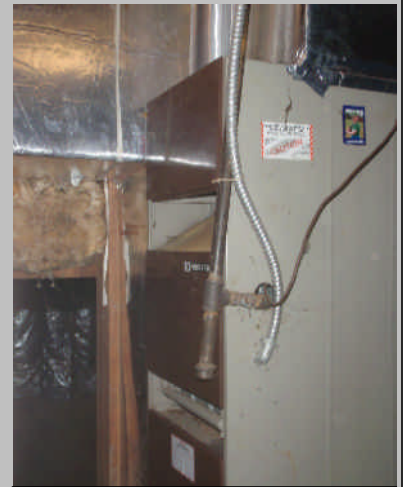
Furnace in crawlspace area.
