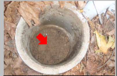
Shut-off covered with dirt.
