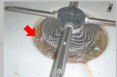
Standing water in Dishwasher.
