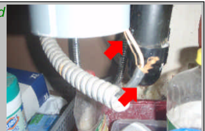
Wire connection missing at base.
