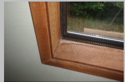
Stains on corners of window sill.
