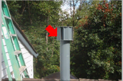
Venting is satisfactory.
